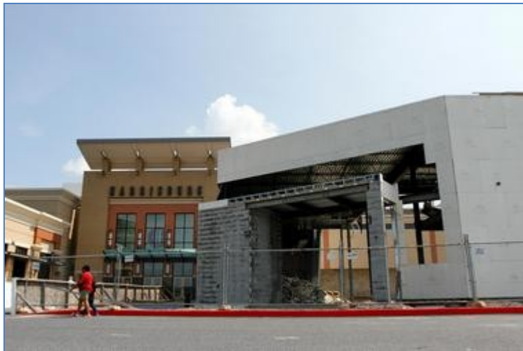
Justin A. Shaw, The Patriot-News, Harrisburg Malls new owners had the partially constructed Sega Sports Bar on the front side of the mall demolished on July 16.
